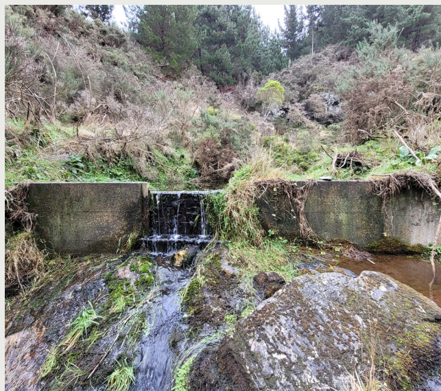
A weir structure designed to prevent salmonids entering a population of threatened galaxiids. Akatore Creek. (photo source: Daniel Jack)
