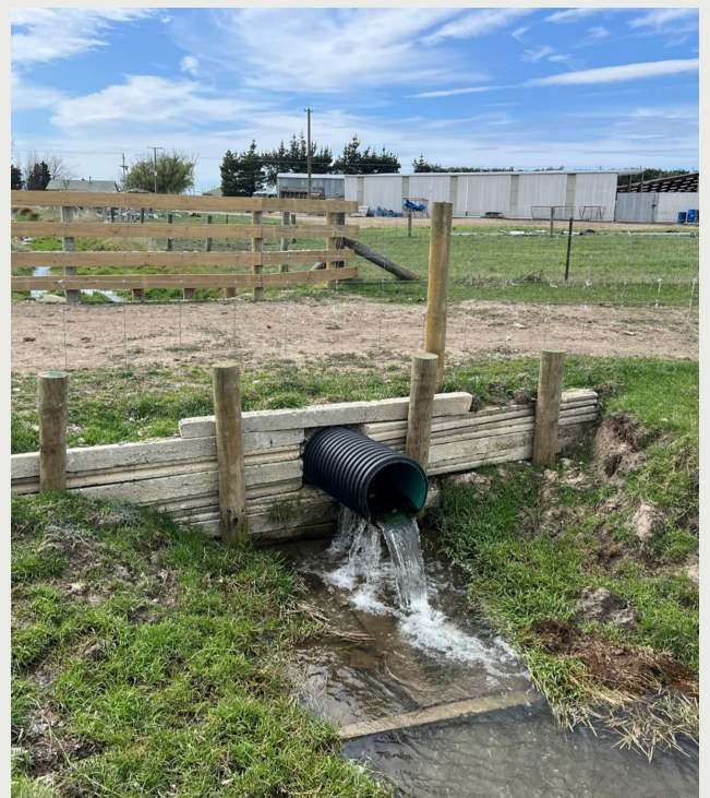
September 2024 Hepburn Road perched culvert
