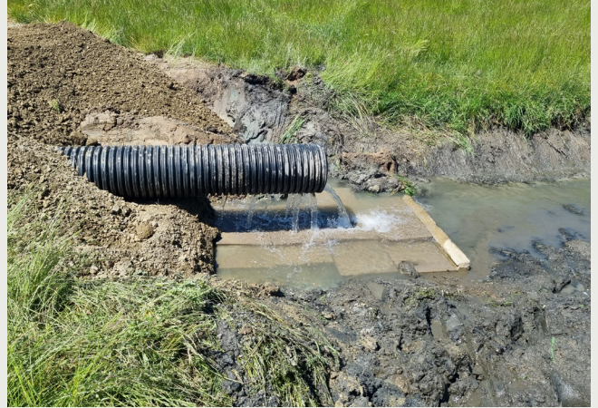
Hepburn Road site pavers in place to avoid the creation of a pool.
